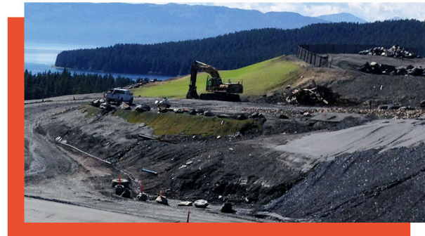
Shown here is an example of a partially reclaimed dry stack tailings storage at Greens Creek Mine in Alaska, which has been operational since the 1980s.
